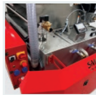
Central switch box with display for controlling all pumps etc.
